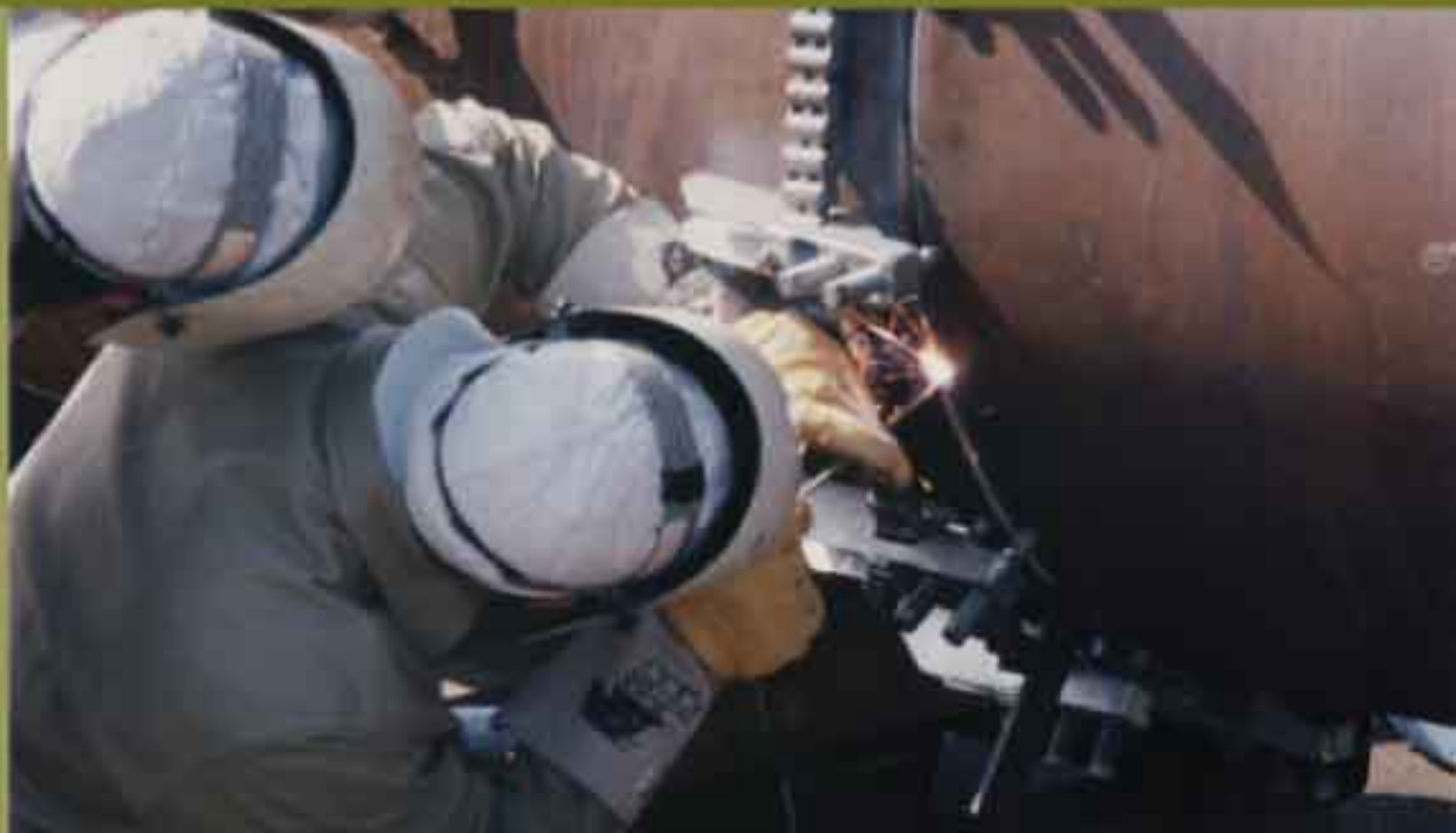
Chain clamp is used to align and hold in position 48-in. pipe for welding.
